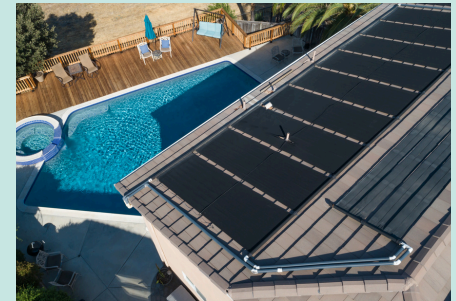
Solar home heating.
