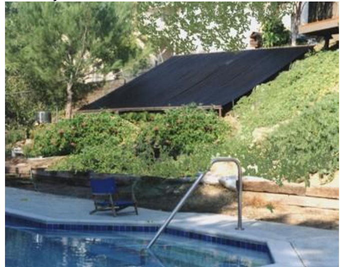
The black panels near the pool side are metallic heat exchangers that absorb solar energy efficiently, and this cost-saving energy to heat the pool.
