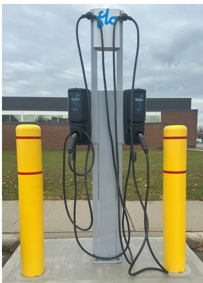
A Level 2 Flo charger installed at The Woodlands High School.
