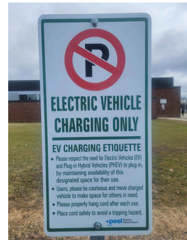
Signage for the charging station installed at The Woodlands High School.
